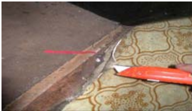
Figure 1 – Asbestos backed vinyl sheet flooring
