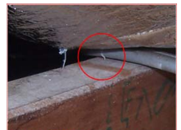
SHOCK HAZARD - Electrical cable pierced by a staple, energising the foil insulation
