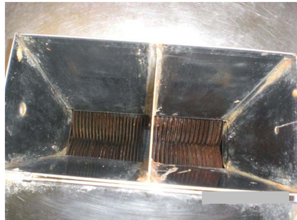
Photograph 2 – The feed hopper showing unguarded access to cutting blades.
