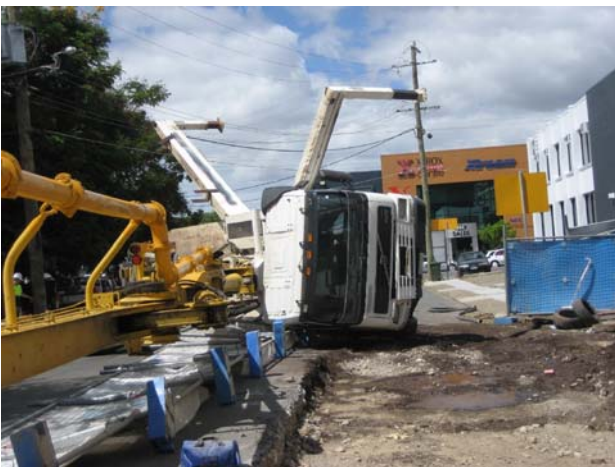
Photograph 1: overturned mobile concrete placement boom
