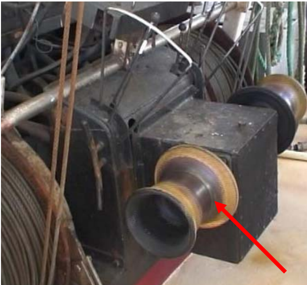
Photograph 1 – Example of an unguarded windlass style winch
